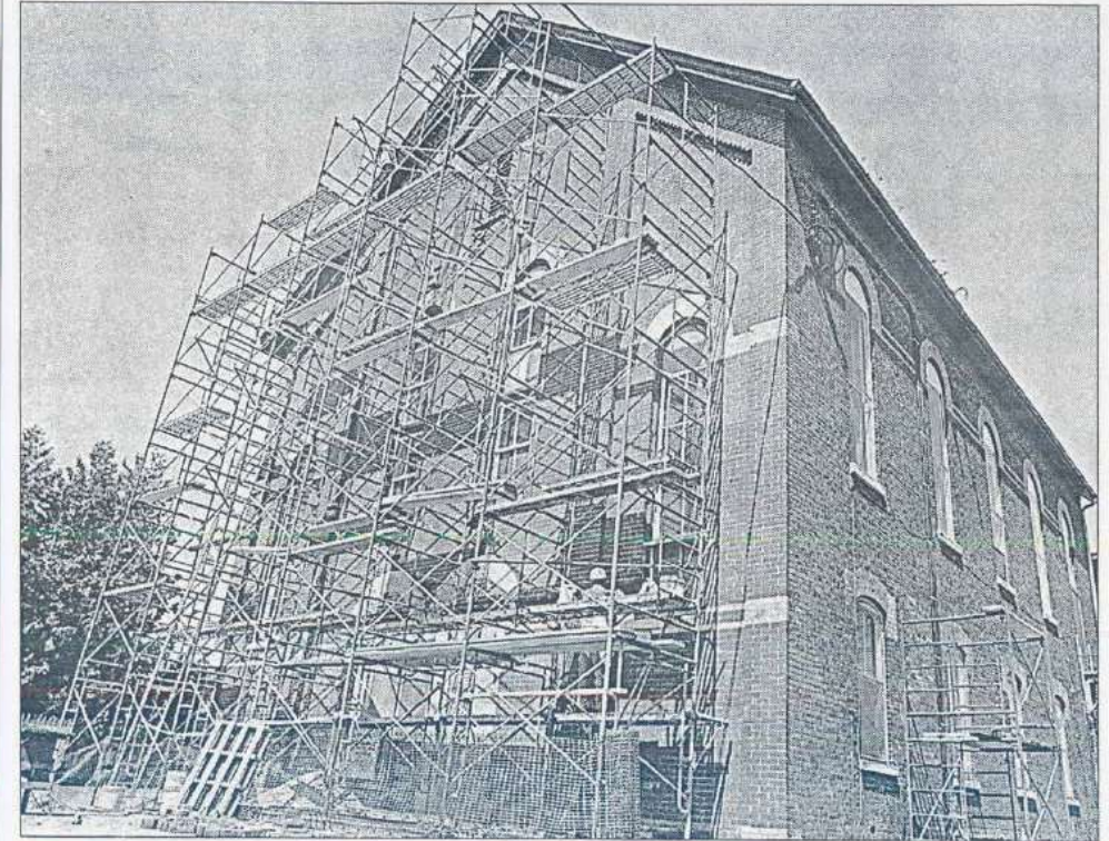
Kevin Morton is a mason working on the exterior reconstruction of the old Cobourg Library on Chapel Street.
